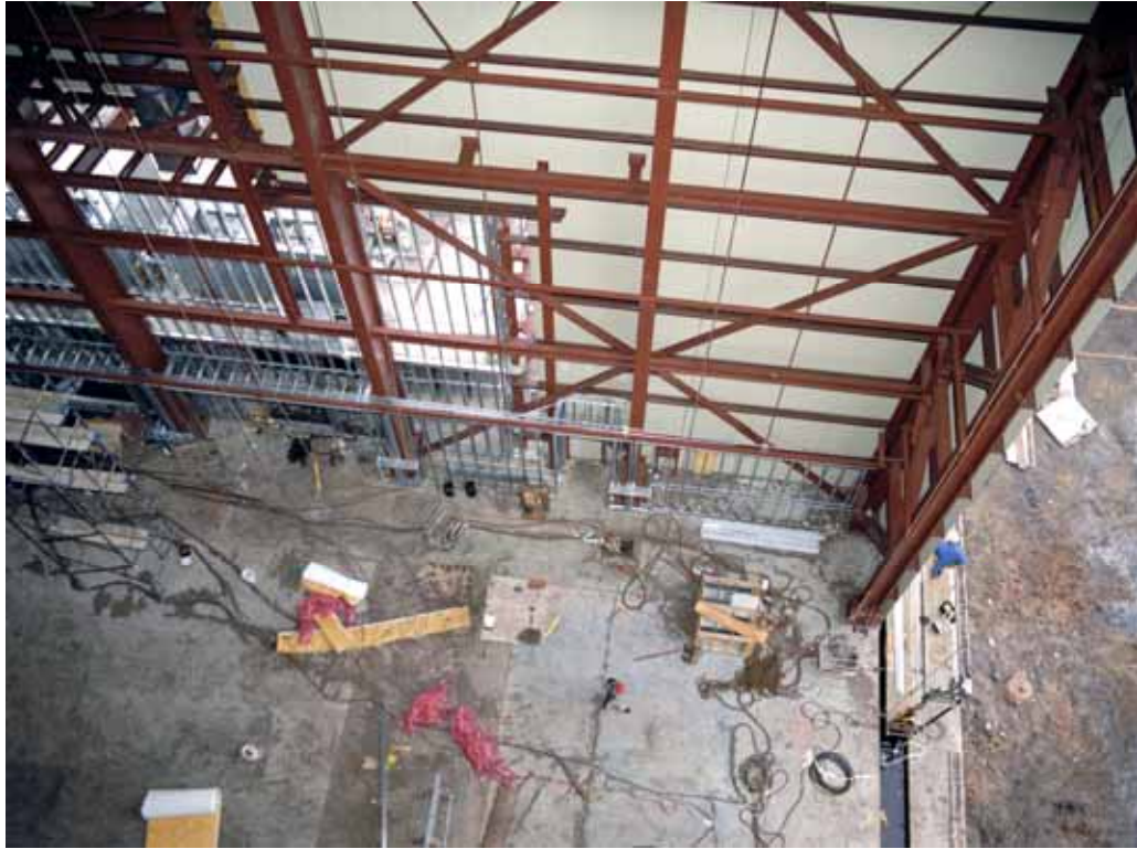
Photo 7. Canister Rotation Facility under construction, 1992. (Source: NASA John F. Kennedy Space Center, 392C-342 FR08)
