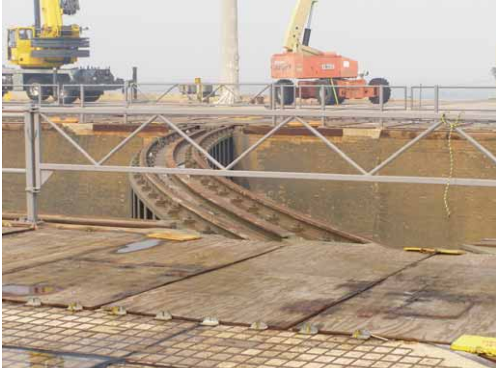
Photo 3. Launch Pad 39A, rail tracks for RSS, facing southwest. (Source: Archaeological Consultants, Inc., 2007)
