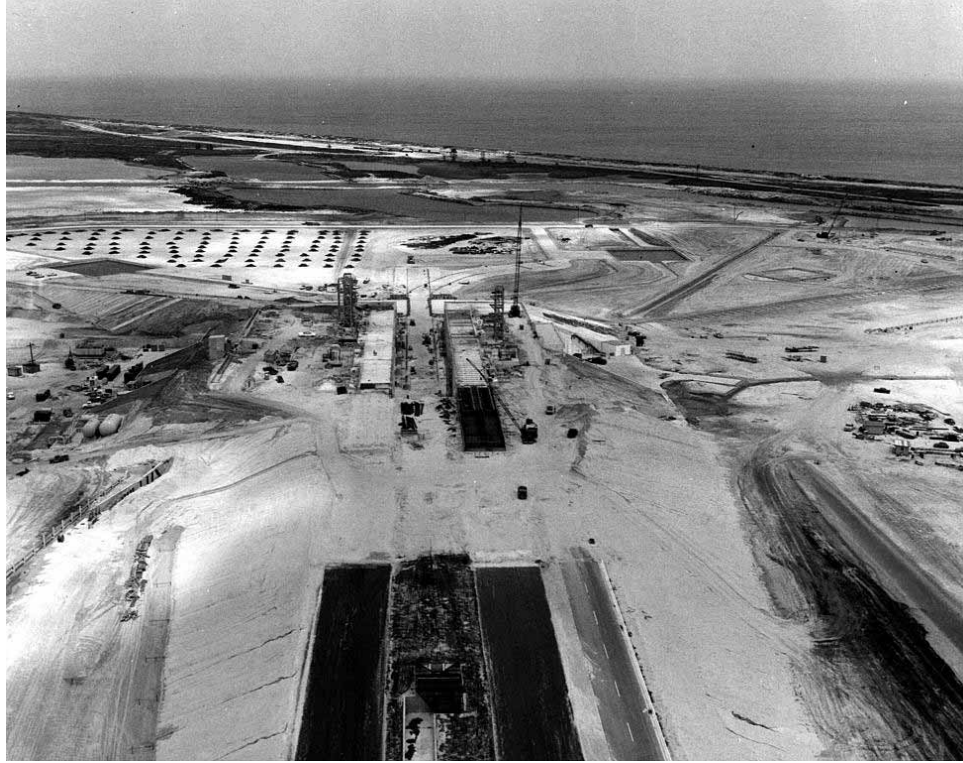
Photo 7. Aerial view of Launch Complex 39A construction, 1965. (Source: NASA John F. Kennedy Space Center, KSC-65C-2305)
