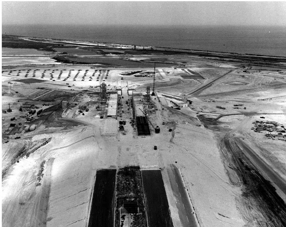
Photo 8. Aerial view of Launch Complex 39A construction, 1965. (Source: NASA John F. Kennedy Space Center, KSC-65C-2305)
