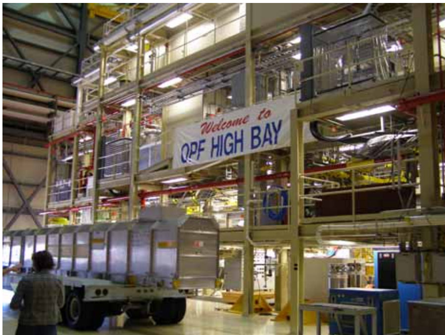
Photo 2. Orbiter Processing Facility High Bay 3, workstand 513, looking northeast. (Source: Archaeological Consultants, Inc., 2006)
