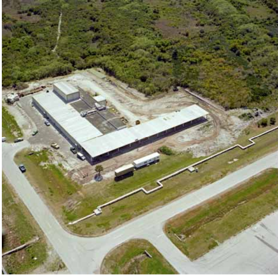
Photo 7. Parachute Refurbishment Facility under construction, 1978. (Source: NASA John F. Kennedy Space Center, 378C-202 FR01)
