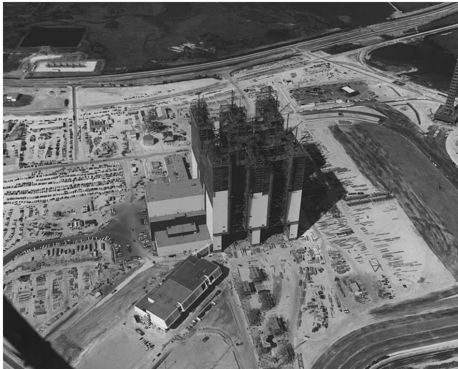
Photo 6. Aerial view of VAB construction, 1965. (Source: NASA John F. Kennedy Space Center, 65C-1458)
