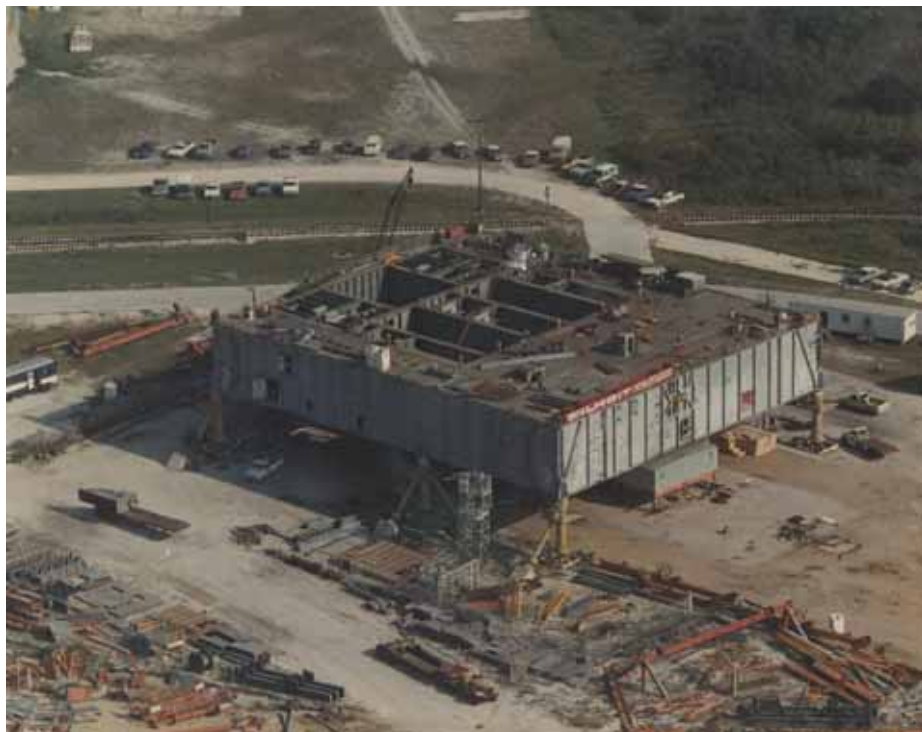
Photo 4. MLP during renovations for Space Shuttle Program, 1976. (Source: NASA John F. Kennedy Space Center, KSC-76C-2754)
