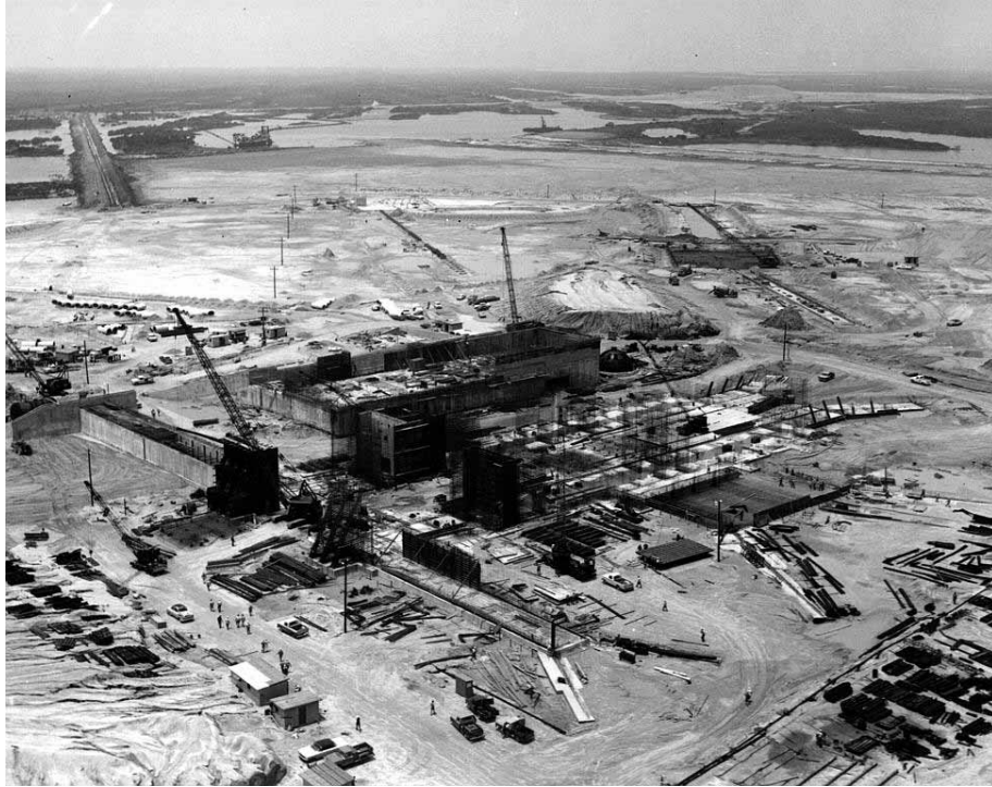
Photo 7. Aerial view of Launch Complex 39A construction, 1964. (Source: NASA John F. Kennedy Space Center, KSC-64C-0027)
