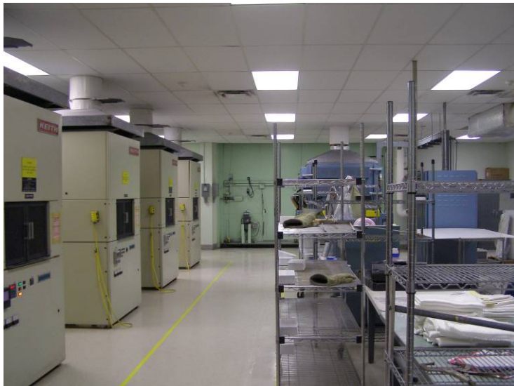
Photo 6.24. Thermal Protection System Facility, heat cleaning room. (Source: Archaeological Consultants, Inc., 2006)
