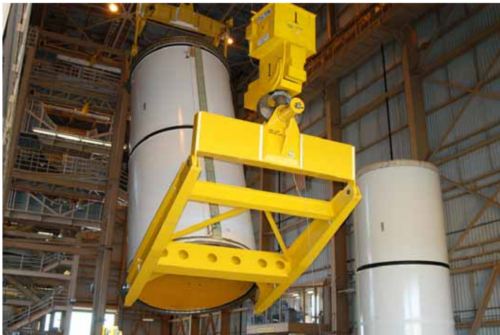
Photo 10. SRB segment being lifted and rotated, 2004. (Source: NASA John F. Kennedy Space Center, KSC-04PD-0058)
