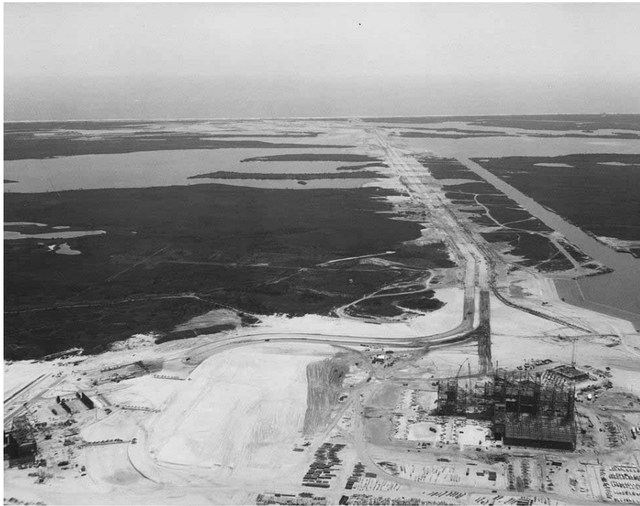
Photo 6. Aerial of VAB, Turn Basin & Crawlerway-early construction phase, 1964. (Source: NASA John F. Kennedy Space Center, KSC-64C-1280)
