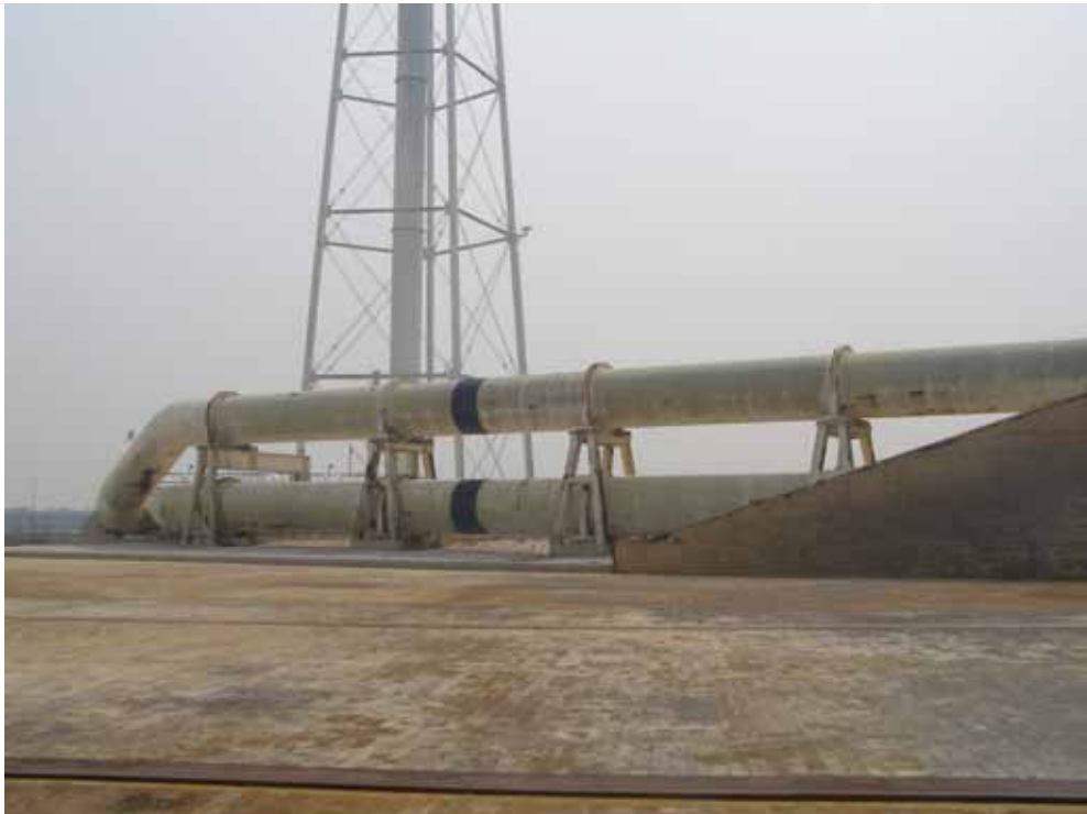
Photo 6. Launch Pad 39B, water suppression system, facing east. (Source: Archaeological Consultants, Inc., 2007)
