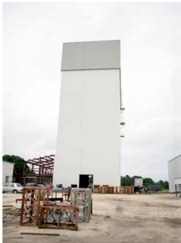
Photo 6. Canister Rotation Facility under construction, 1992. (Source: NASA John F. Kennedy Space Center, 392C-341 FR04)
