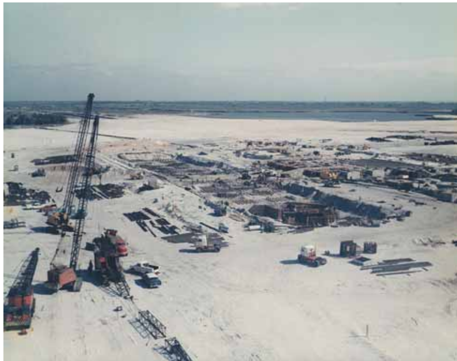
Photo 4. Aerial view of VAB foundation construction, 1964. (Source: NASA John F. Kennedy Space Center, 64C-0276)
