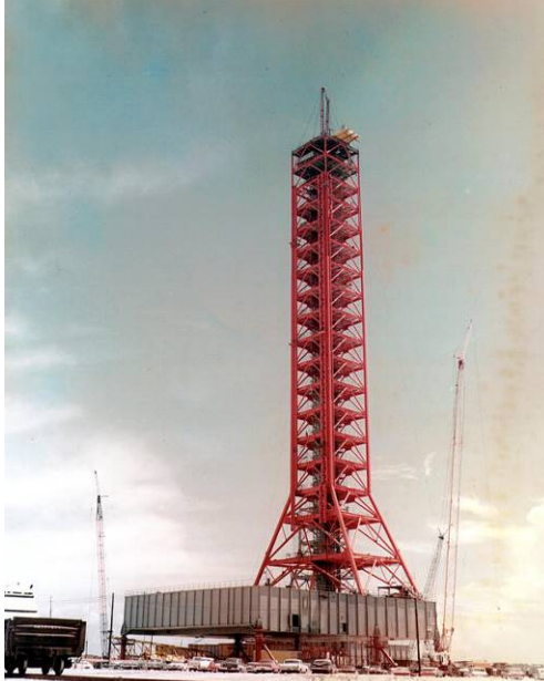
Photo 6.45. LUT and mobile launcher construction, August 1964. (Source: NASA Kennedy Space Center, KSC-64C-3077)
